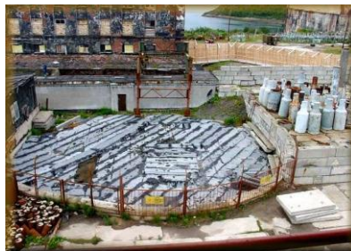
Figure 8.2. View of the concrete roofing of the DSU at STS in Andreyev Bay
