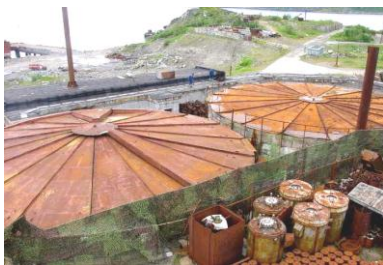
Figure 8.1. View of the roof of the DSU at STS in Andreyev Bay
