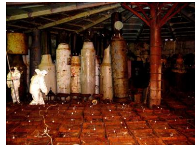
Figure 8.3. Containers installed in one of DSU facility
