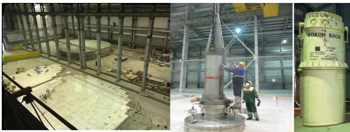
Technological hall of Building 153 (in the foreground - DSUs 2A and 2B, in the background - DSU 3A), Reloading container for SFA, Transport package container (source: SRC-FMBC).
