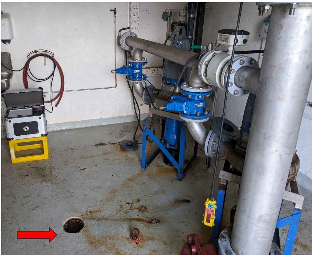
Figure 7. Dwarf 100x9 portable air sampler in the pump station at Breivika. The red arrow indicates the opening in the floor (14.5 cm in diameter) to the sump where wastewater collects before it is pumped further to the Breivika WTP through the pipework visible on the right-hand side (Photo DSA).
